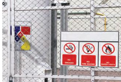
Electronic Devices Installed Within Explosive Environment
