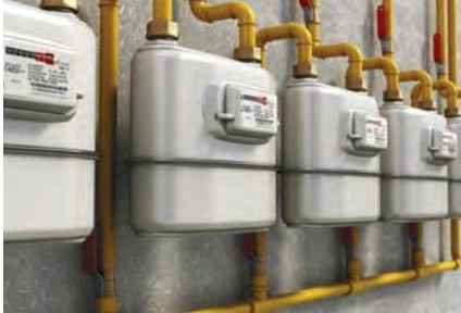
Gas Meter & Gas Distribution System
